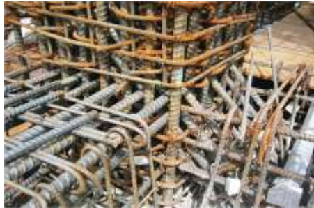
Fig. 2 Congestion at the Beam-Column Joints (ref.: www.concreteconstruction.net )
